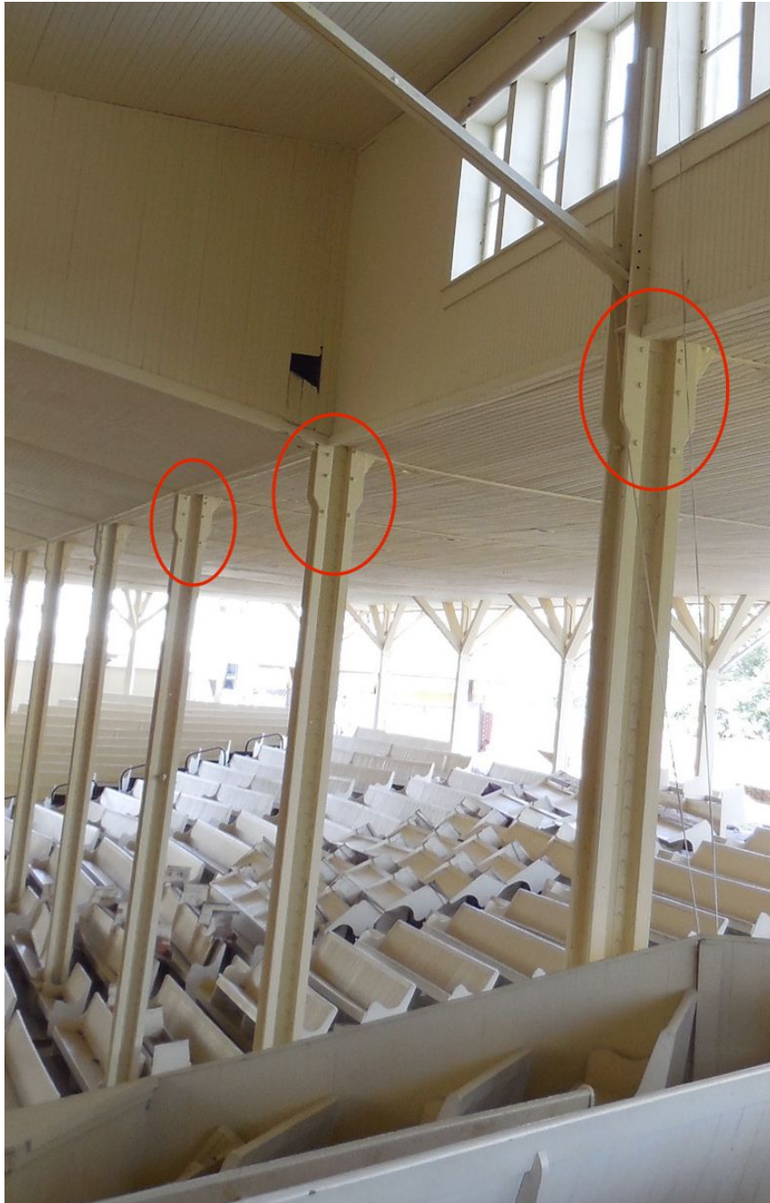
Image 5. Existing columns. Circled in red increase of reinforcement at the point of hishest stresses.
